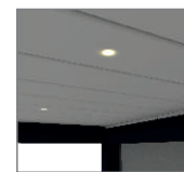
LED lighting - spotlights
